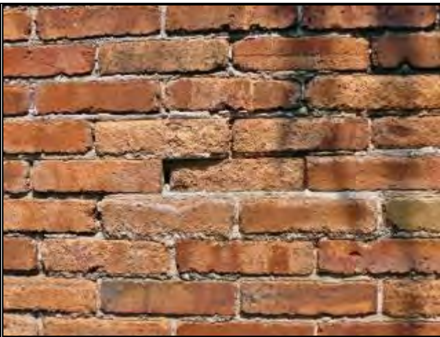
Photograph 121: Spalling Brickwork, Planetree Road
