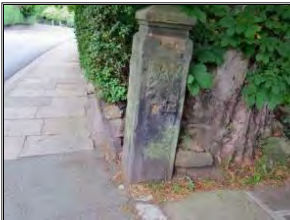
Photograph 33: Low Wall pushed out by Overgrown Hedge
